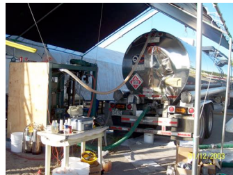
Static resin mixer connected to one of the 8 tankers of resin required to complete the Wetout of the liner
